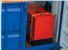
Storage Container & Generator
