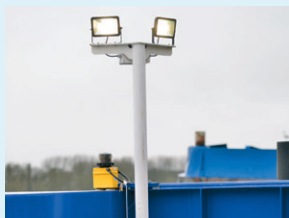
Floodlight and mast
