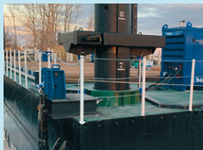
Railing sceptors and steel wire
